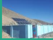
A solar-powered water supply network handed over in Mirzaka district ...
